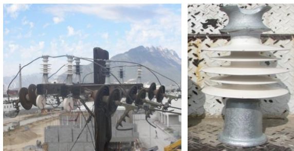
Fig. 1. Silicone rubber insulators in a 13kV distribution line and a close-up of one insulator
