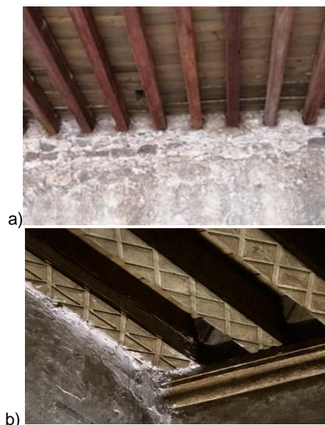
Fig. 6. Timber joist mezzanine system, a) beams supported directly on the masonry wall, b) beams supported on a trailing beam in the chancel area. Images taken from [21]
