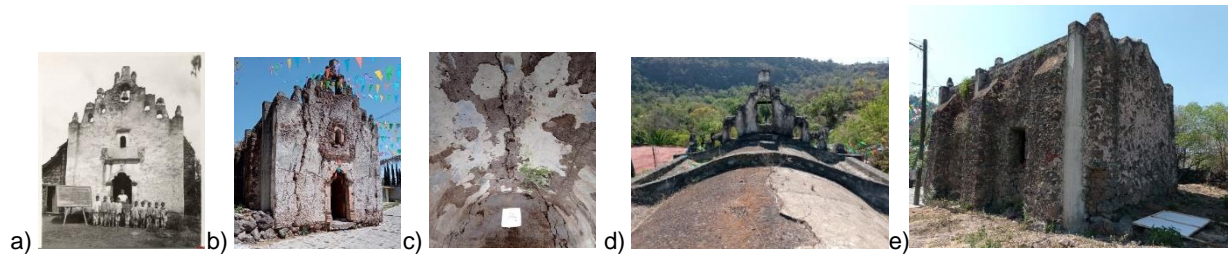
Fig. 13. Chapel of Santa Catarina, a) facade preserved in the 20th century, b) present state of the facade, c) current condition of the interior of the vault, d) side wall and buttresses, e) present state of the exterior of the vault. Images taken from [3,24].
